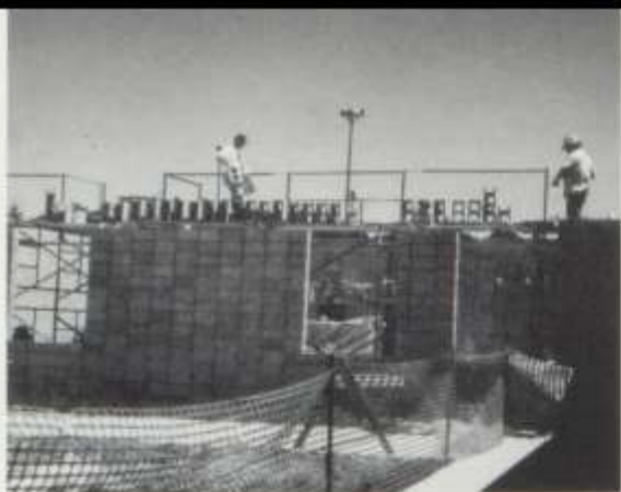
Starting on the construction at the back of the school are the construction workers. The school is adding on a Special Ed. Department, an artroom, and an extra classroom.
